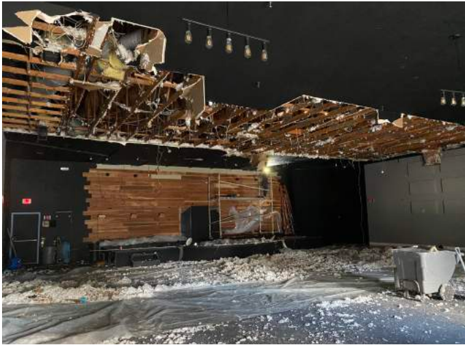
Auditorium 24 hours after the incident
